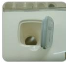
Water supplyment for humidification
